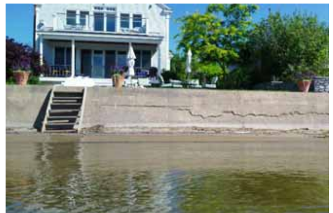
The push and pull of ground water from the landside plus waves from the lakeside, rock sea walls back and forth leading to cracks like this one. Cracks can be seen in scores of sea walls around the lake. Photo by Mike Winslow.
