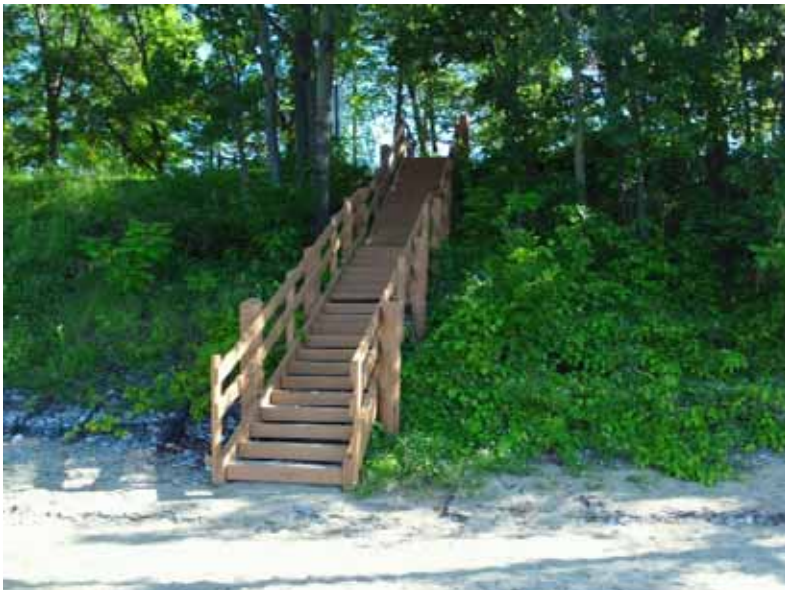
A designated staircase limits trampling of vegetation and preserves soil on slopes. Note too, gabions to left and right of staircase provide protection from erosion, but allow vegetation to grow through the wires. Photo by Mike Winslow.
